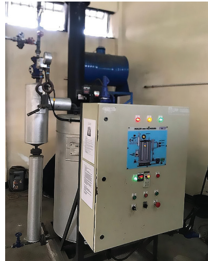
Fig. 2. Boiler type TWA 300 kg/hours
